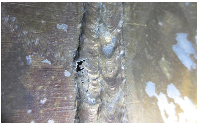
Fig. 3 CORRODED 2205 WELD DUE TO UNDER-ALLOYED WELD METAL
